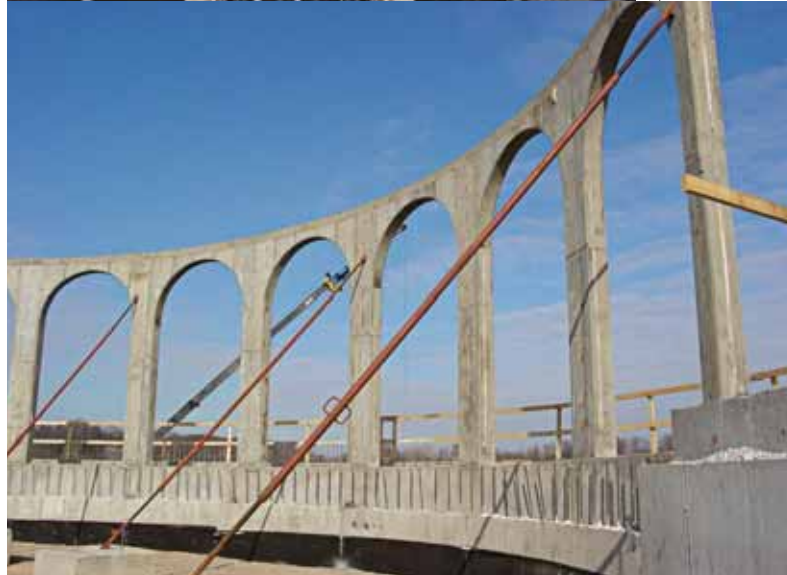
These before-and-after construction shots show self-consolidating concrete placed in a tall and slender pour with congested reinforcing steel.
