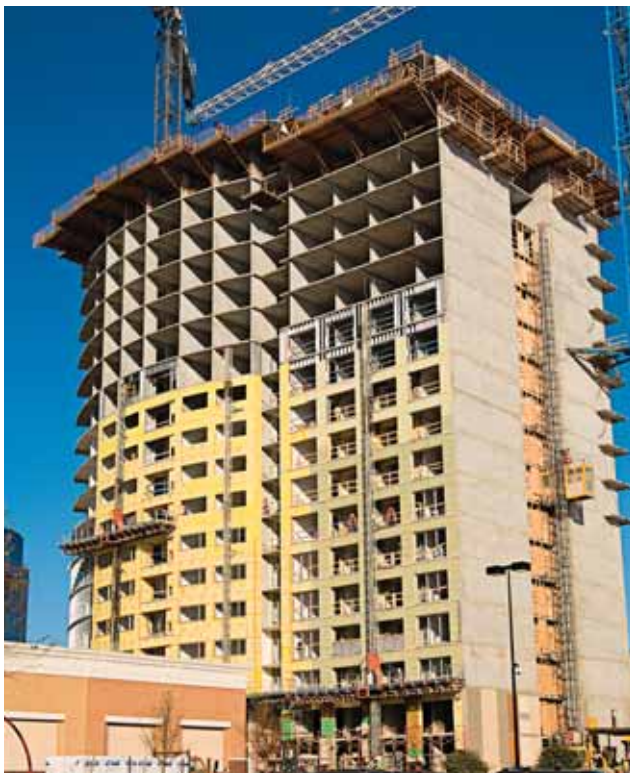
Air and moisture barriers are critical to building envelope design. They help reduce risk of excess moisture and improve HVAC efficiency.
