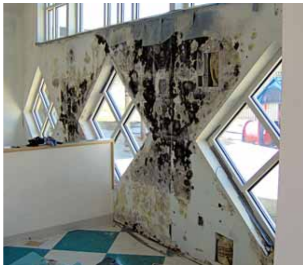
Example of building envelope failure combined with a vapor barrier on the interior face of the walls covered with vinyl wallpaper.
