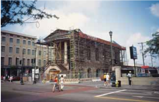
A stucco veneer at Charleston's Market Hall, original constructed in 1841, is being repaired.
