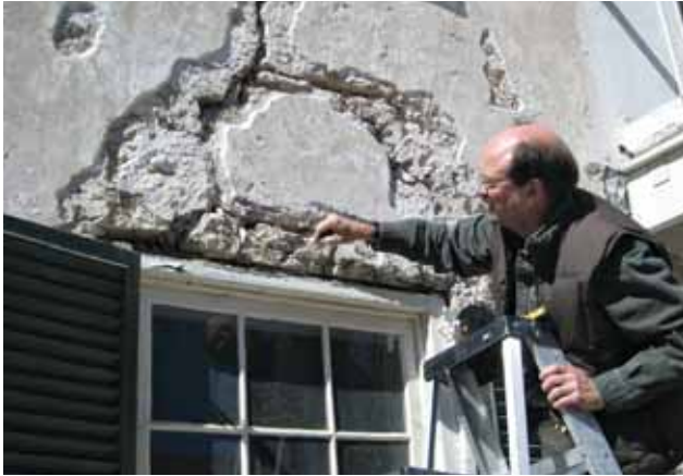
A coquina stone façade on a 1797 Spanish Colonial structure in St. Augustine, Fla., is inspected prior to patching.
