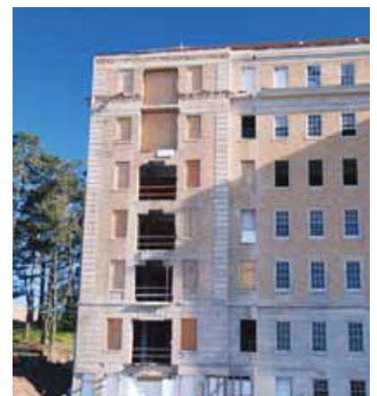
Façade restoration in progress at the historic PHS Hospital. Built in the 1930s, the hospital is being converted into a 22,000-sf apartment building.
